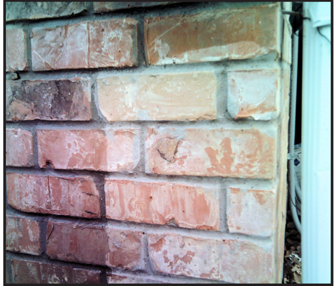
We sprayed this brick wall with water after treating part of it with WB RAINSEAL. See the difference?
